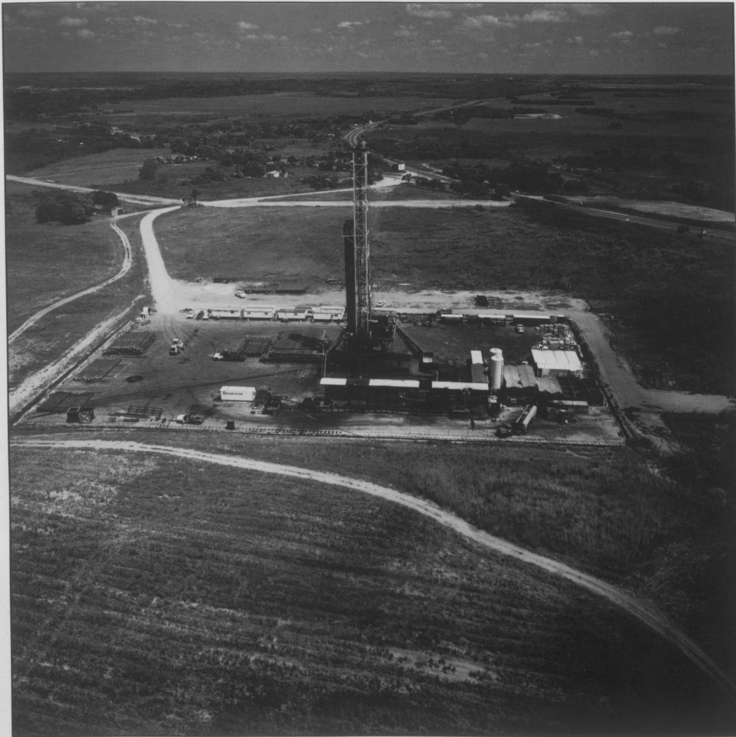
Lagoven inaugurated a water injection project in the El Furrial Field, to improve crude oil recovery.
