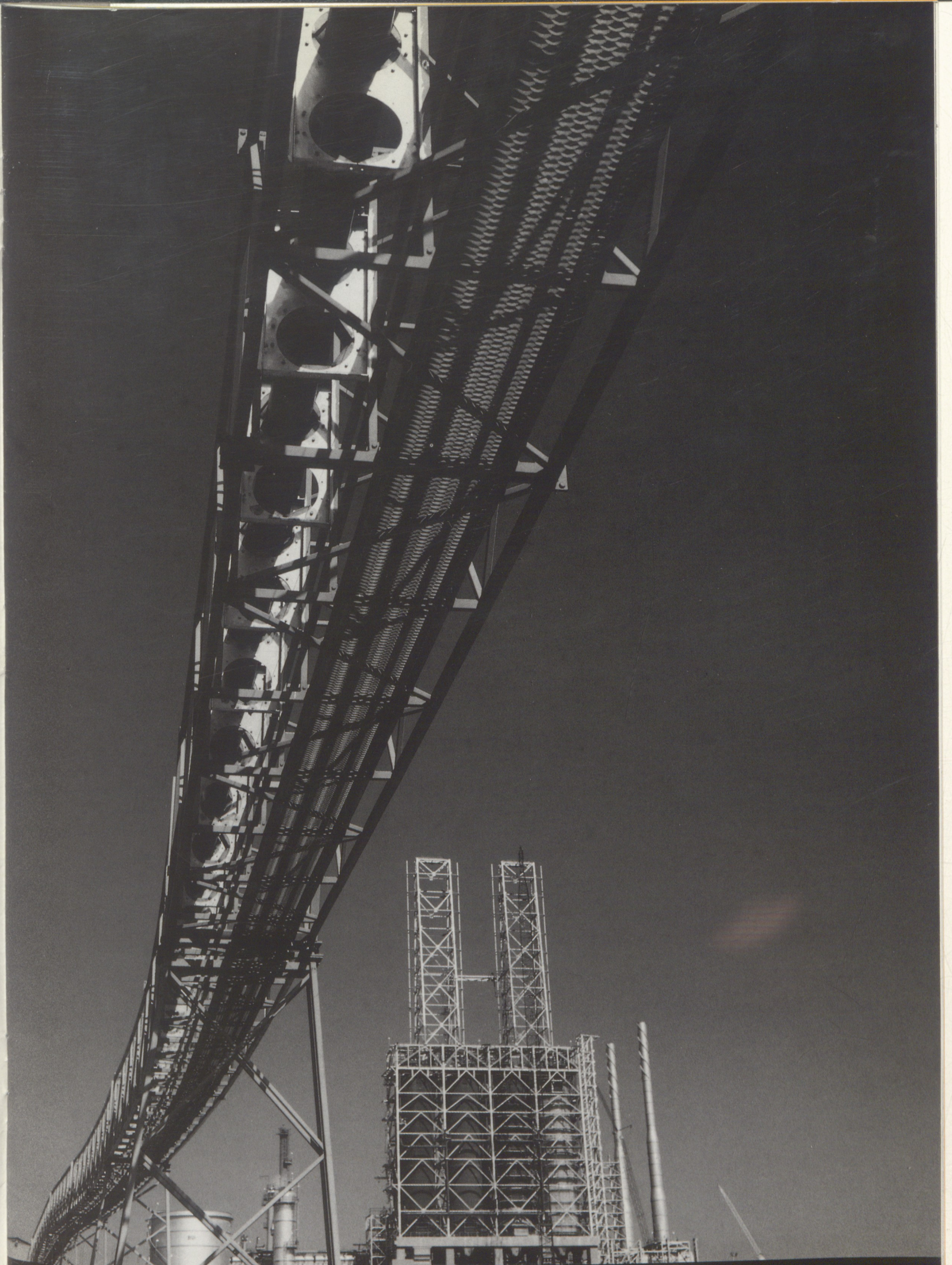
According to plan, progress was made on construction of a delayed coker plant at Amuay Refinery
